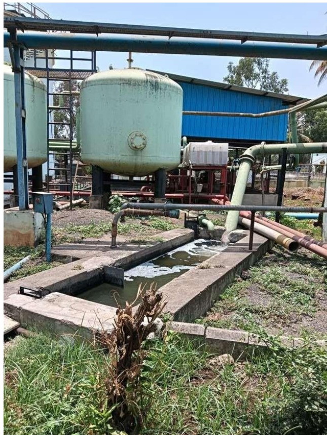
Fig no. 2 Effluent treatment plant
