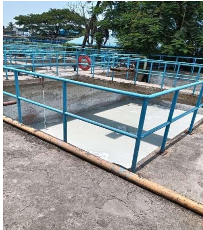
Fig No.1 Sewage treatment plant
